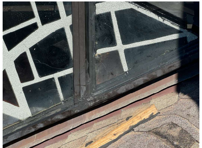
Photograph 10. Most of the protective glass frame joints have been sealed on the west upper clerestory; however, the sealant was not cleanly applied at all locations
